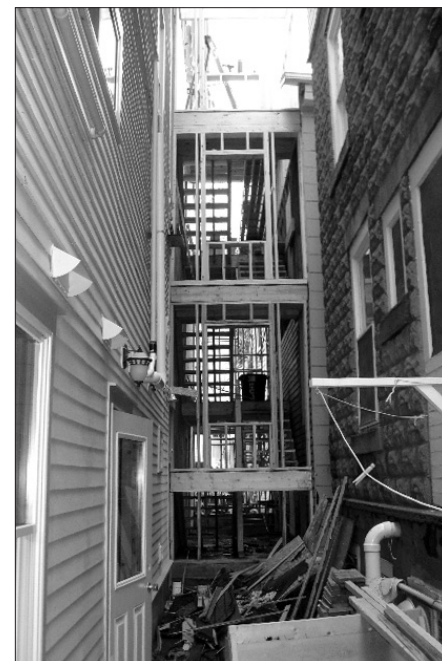
The new elevator tower framed between the Bird-Werner and the Westervelt buildings. The Shaw building is in the left foreground.
